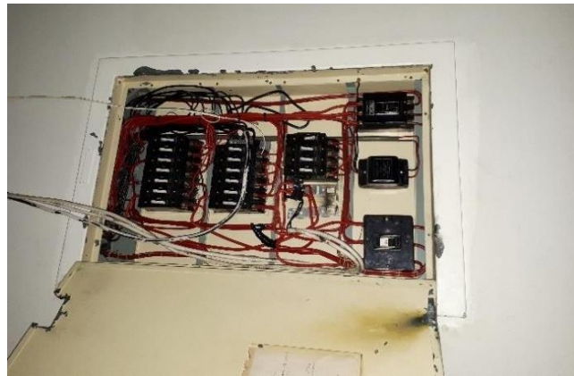
Photo 4: Informal electrical connections
