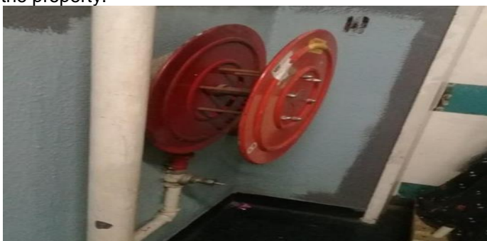
Photo 2: Detective fire hose reels
